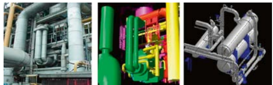
Fig. 3: Petrochemical installation of the FPSO
